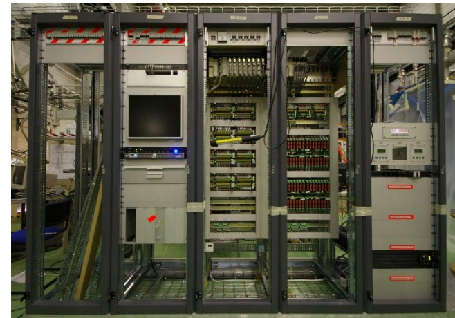
ArDM control system
