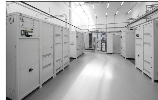
SOLEIL ramped power supplies for booster magnets
