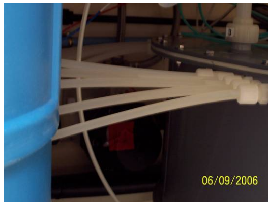
Figure 10: The tank is in PVCC (grey) and coil in PVDF.
