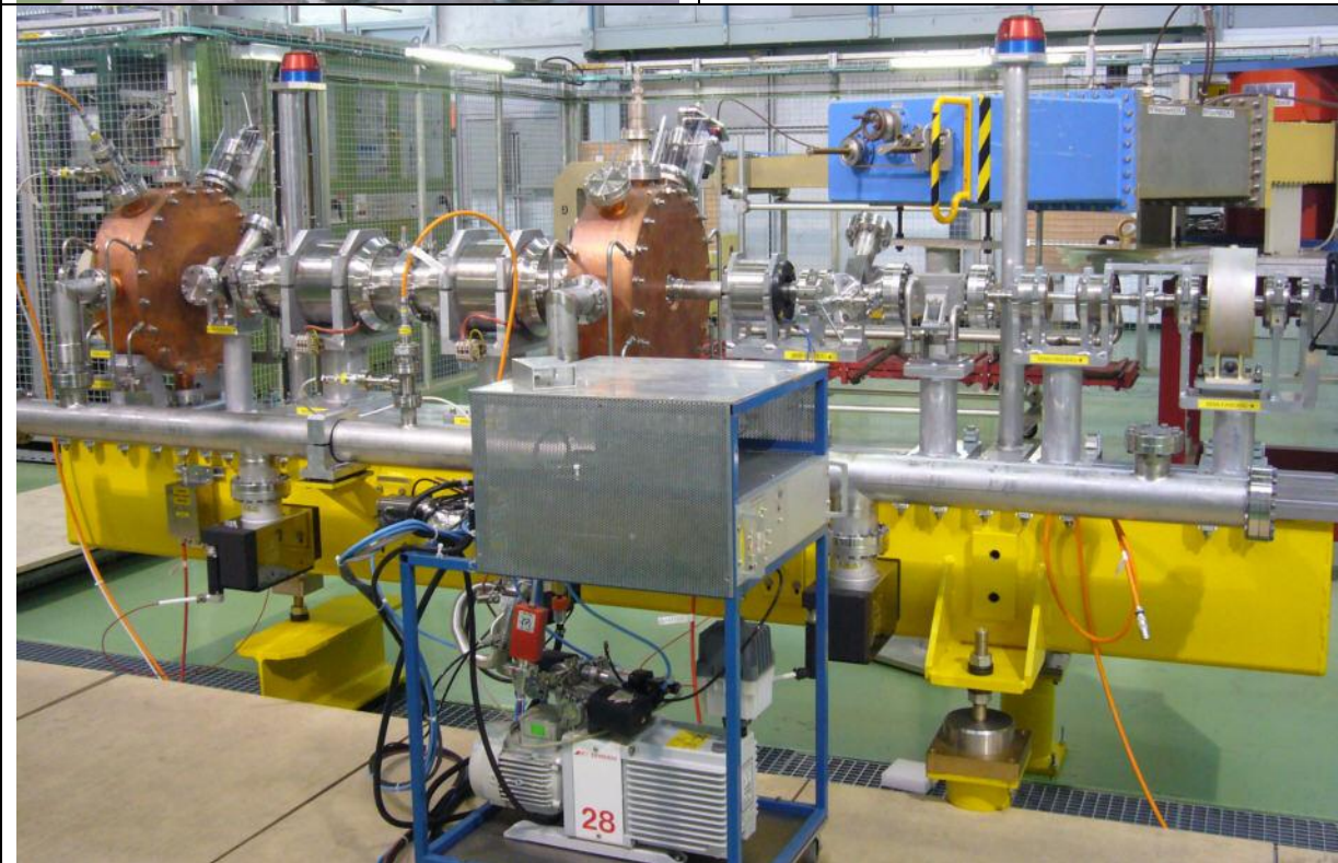
View of the line assembled and under vacuum.
