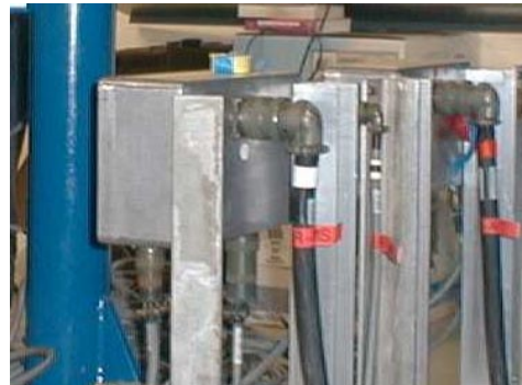
Figure 5 : Connection boxes on the upper ring
