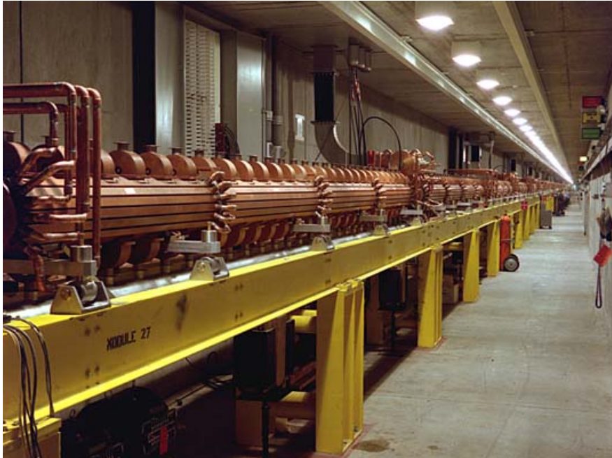
Figure 3-2 – The LANSCE Coupled Cavity Linac (CCL), high-energy section of the 800 MeV Los Alamos proton linac.
