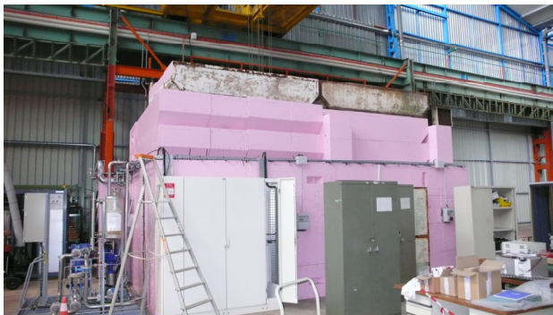
FIGURE 6. The concrete shielding installed in our laboratory.
