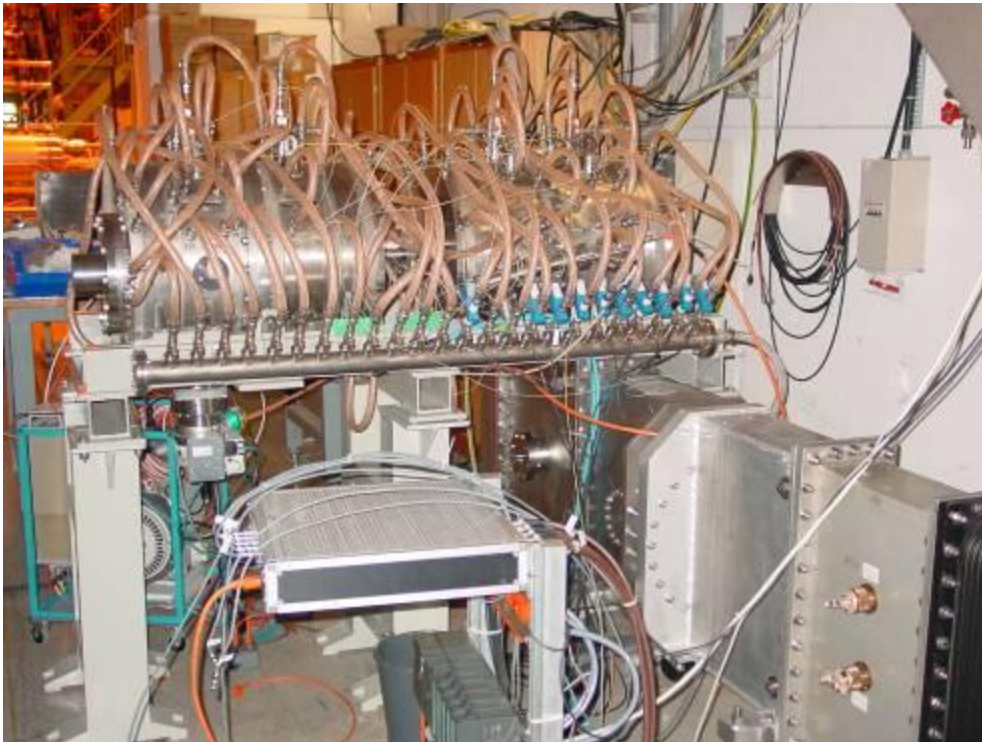
Figure 12 ISTC CCDTL prototype installed inside the bunker at SM18
