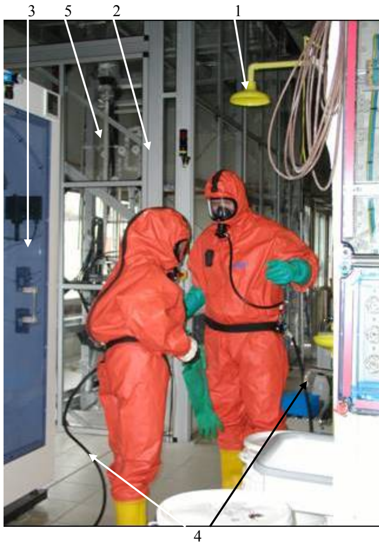
Figure 14 A DESY crew prepares themselves for the repair of the heat exchanger unit. The crew is protected against hazards of the acid and gas from the EP acid by safety overalls (Dräger type Workmaster®)
