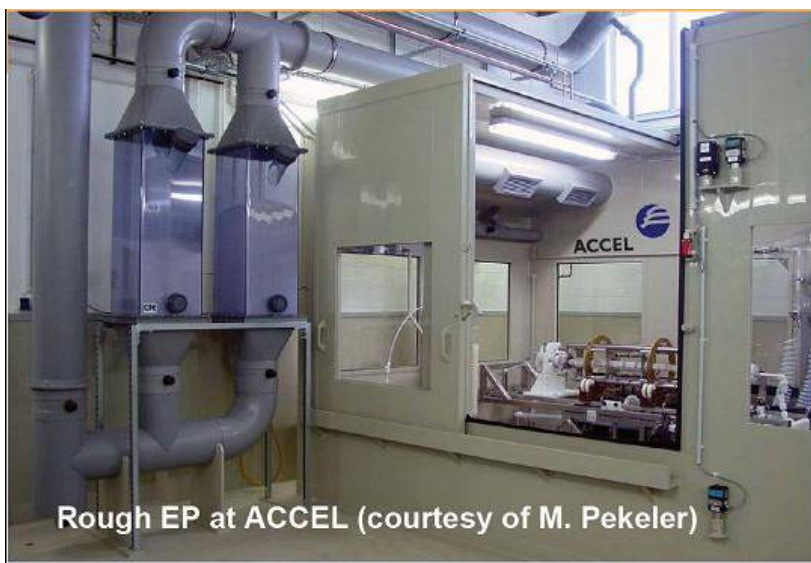
Figure 14 EP installation at ACCEL Company
