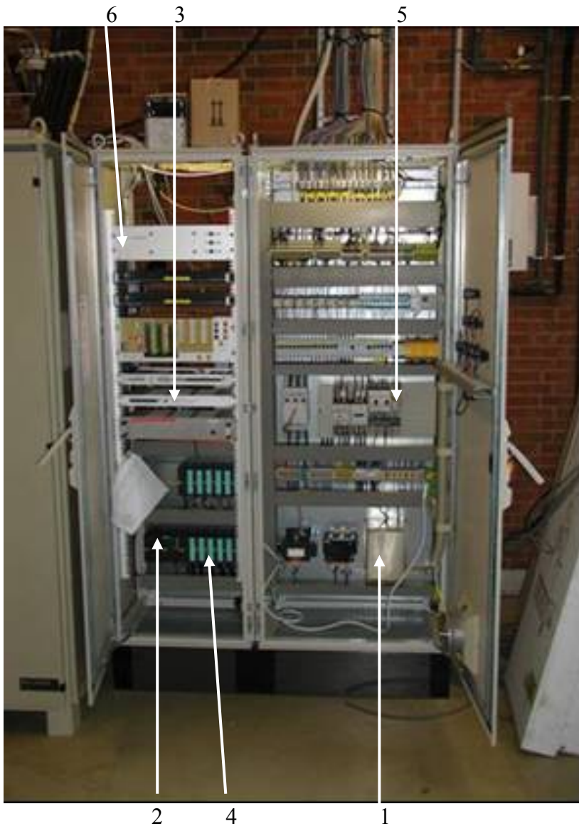
Figure 13 View on to the control cabinet (left side) and power distribution panel (right side) of the DESY EP infrastructure.
