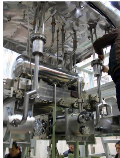
Installed in the Cryomodule
